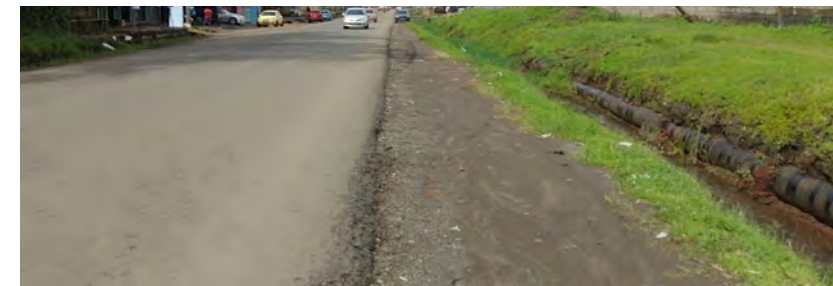
EXPOSED WATER SUPPLY PIPE ALONG MWIKI KASARANI ROAD
