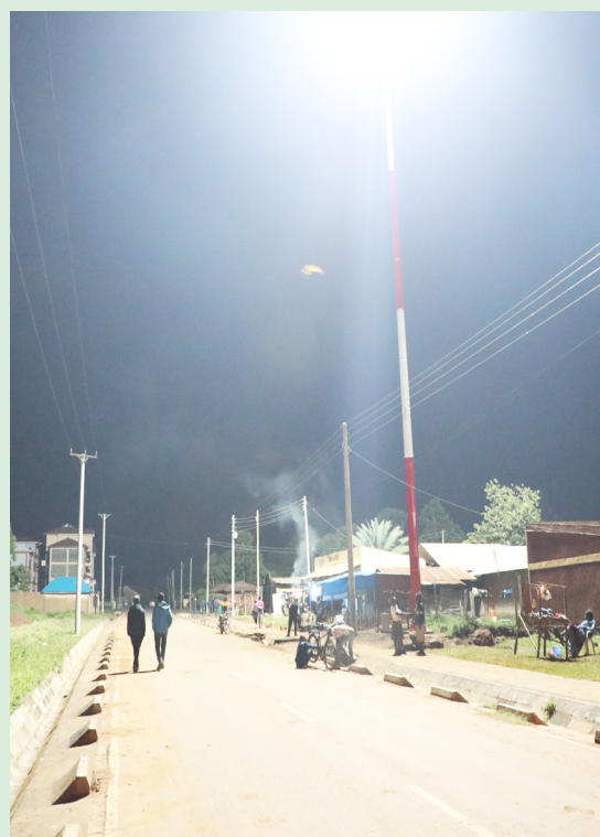
Completed high Mast Security Lights at one of the informal settlements in Bungoma town.
