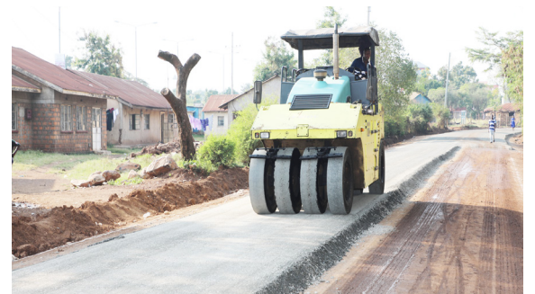
Ongoing roads improvement works in Manyatta A informal settlement in Kisumu County
