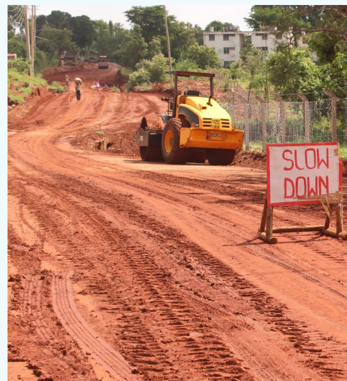
Upgrading of Upper Kariokor-Aseko-Mlekenyi road to bitumen standards in Taita Taveta County by KISIP2
